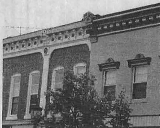
The cornice at left appears to be original. The cornice at right is a reconstruction that seems accurate on the whole. Always base reconstructed ornament on photographic evidence rather than conjecture. For instance, the semicircular elements over the window hoods on the right are questionable.
